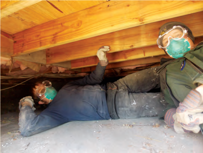
From left, Phil Bartoletti of Penn State DuBois, and Andrew Newswanger of University Park, work in a crawl space under the Nassau Christian Church in Baldwin, New York.
